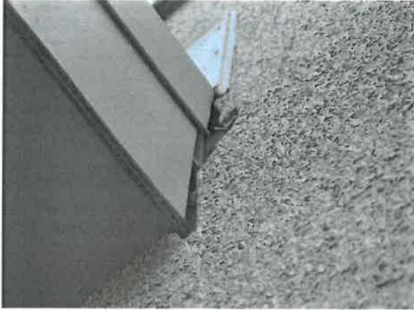
Figure 3-1 Missing Stucco at Canopy to Wall Location
