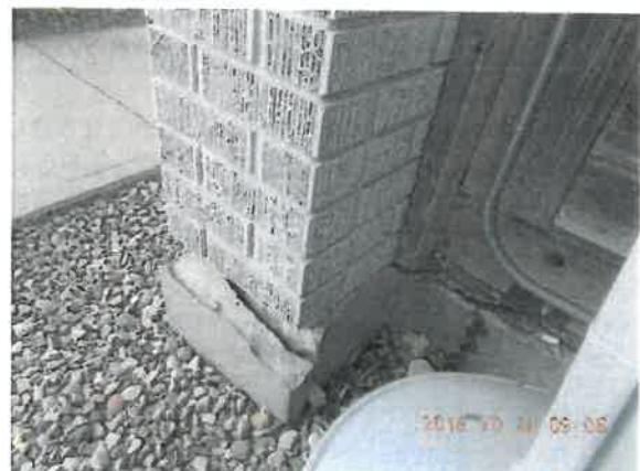
Figure 4-2 Example of Spalled Termination End of Strip Footing Near Main Entrance
