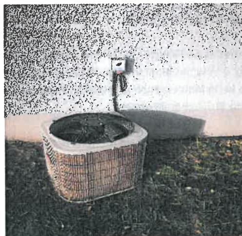
Figure 5-15 Condenser Unit Standing On Grade
