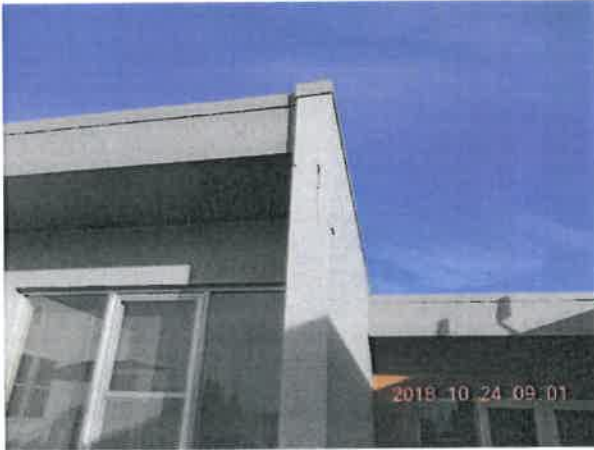
Figure 4-12 Viewing Split Face of End Unit of Bond Beam at SE Corner of Chamber
