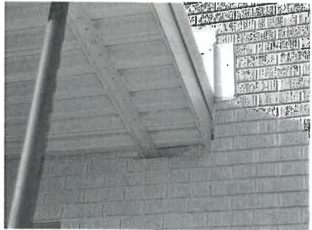
Figure 3-4 Broken Face Bricks Under East Exit Canopy
