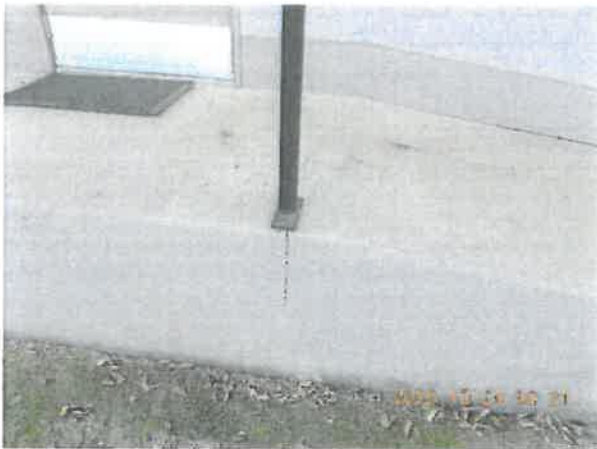
Figure 4-24 Viewing Vertical Crack under Column on North Apron of North Wing
