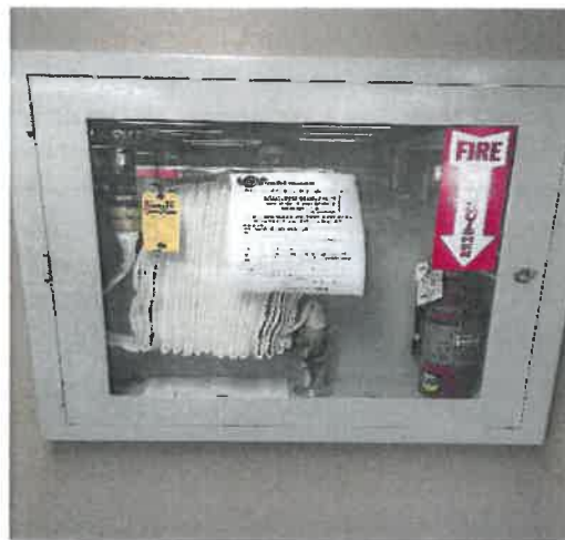
Figure 5-16 Fire Hose Cabinet with Fire Extinguisher
