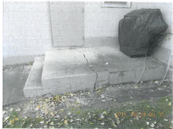
Figure 4-25 Viewing Wide Cracking in West Entrance of North Wing
