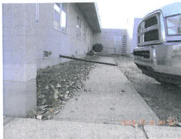
Figure 2-9 Viewing West Sidewalk
