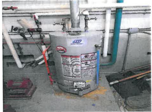
Figure 5-2 Domestic Water Heater
