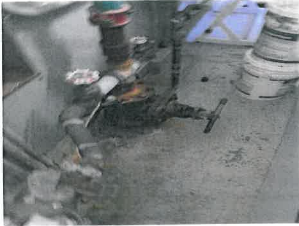
Figure 5-1 Incoming Water Service
