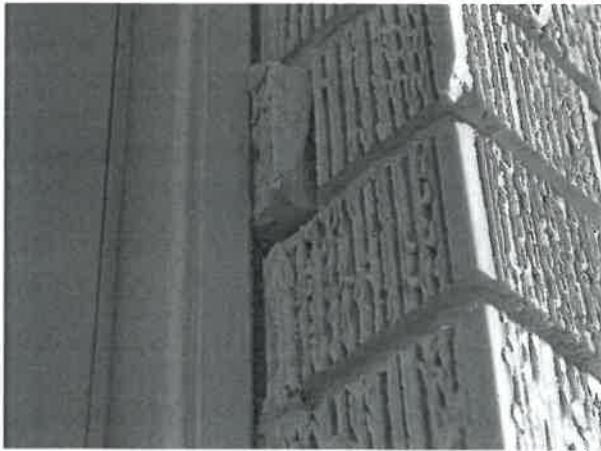
Figure 3-3 Broken Face Bricks at South Exit Door Opening
