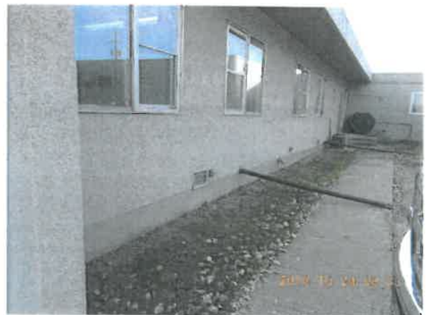
Figure 2-6 Viewing Ponding Location at West Wall
