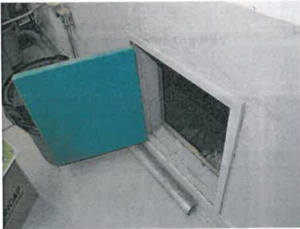
Figure 3-40 Access Door and Frame to Crawlspace in Mechanical Room Not Fire-Rated
