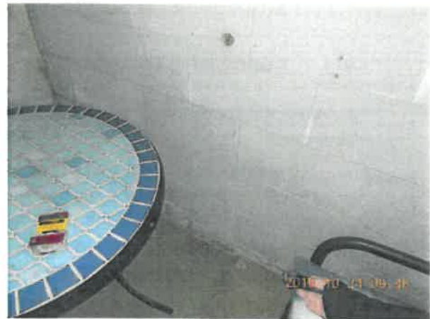
Figure 4-19 Viewing Penetration with Vermiculite Fill Being Expelled in the Original Incinerator Room
