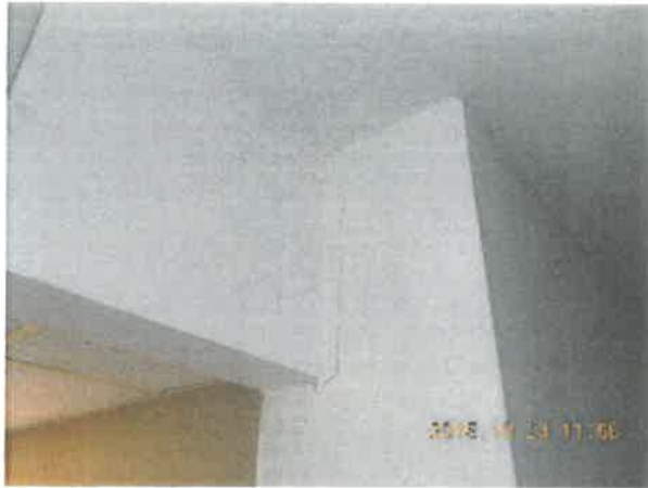
Figure 4-10 Viewing Cracking at Beam Bulkhead
