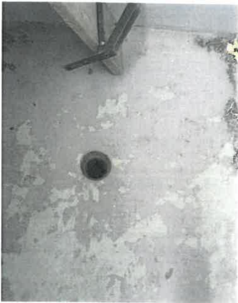
Figure 5-6 Floor Drain Missing Grate
