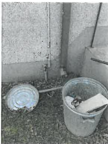
Figure 6-5 Cover Plate Missing on Conduit Junction Box
