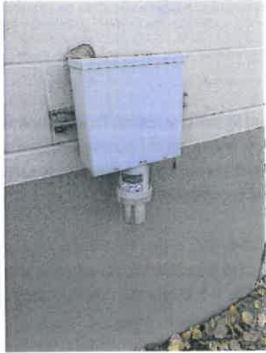
Figure 6-1 Exterior Generator Connection JB
