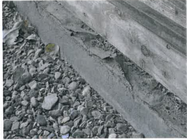
Figure 3-8 Exposed and Deteriorated Building Paper, Missing Base Flashing
