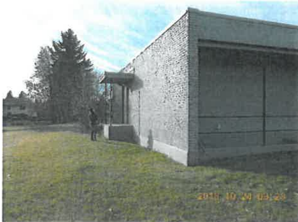
Figure 2-3 Viewing Negative Grading at East Wall
