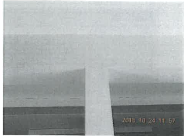
Figure 4-11 Viewing Cracking at Column Connection to Beam and Screws Pushing Out at Ceiling
