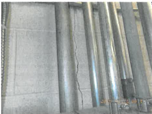
Figure 4-18 Viewing Wide Crack in Interior Face of North Wall of Boiler Room
