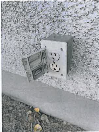
Figure 6-7 Missing Weatherproof Insulation
