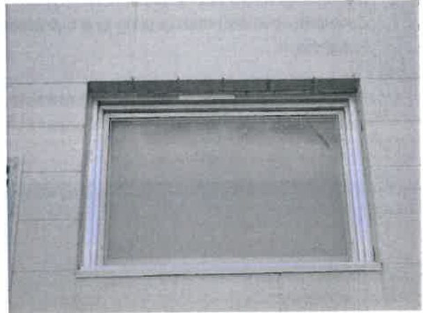
Figure 3-20 Broken Sealant Around Fixed Aluminium Window Frames
