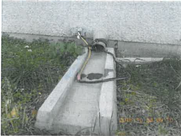
Figure 6-9 Exterior Heat Trace
