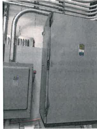
Figure 6-2 Black Substance Observed on Utility Fuse Box
