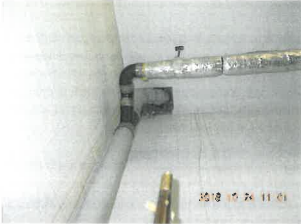
Figure 4-4 Viewing Staining on Wall in Boiler Room
