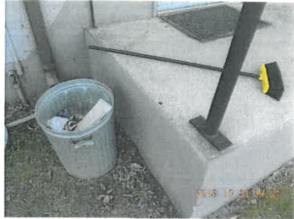
Figure 4-23 Viewing Horizontal Crack on North Apron of North Wing
