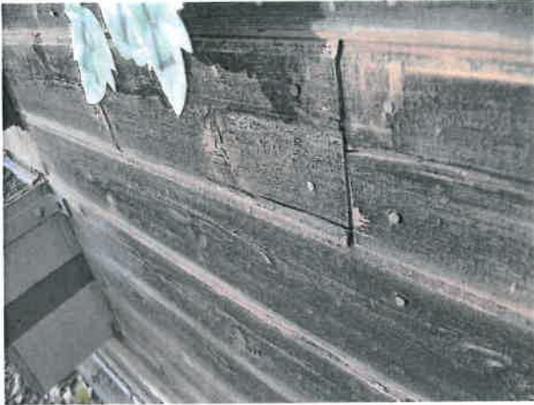
Figure 3-5 Discoloured and Deteriorated Wood Siding
