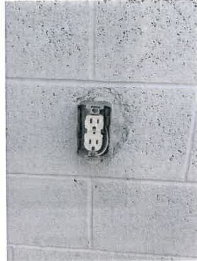
Figure 6-8 Exterior Receptacle Cover Missing
