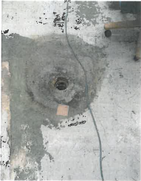
Figure 5-5 Floor Drain Missing Grate
