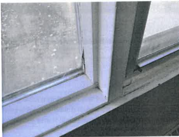
Figure 3-21 Condensation Between Fixed Window Panes, Broken Sealant at Bottom of Vertical Lift Insert
