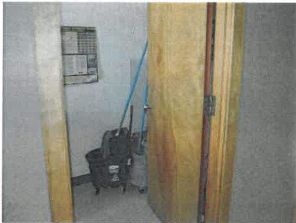
Figure 3-34 Wood Door and Frame to Janitor Room Not Fire-Rated
