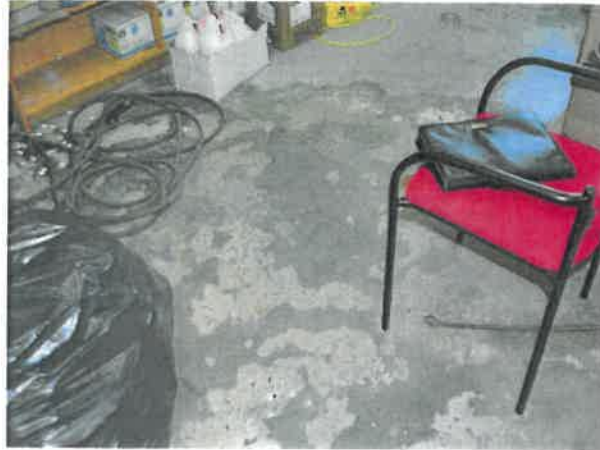
Figure 3-31 Concrete Scaling in Mechanical Room
