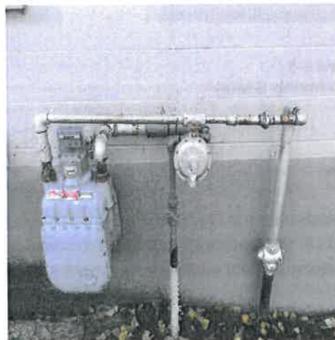
Figure 5-8 Gas Meter and Regulator
