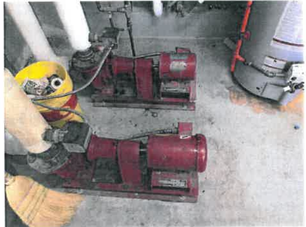
Figure 5-10 Heating Water Pumps
