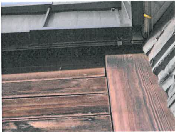
Figure 3-7 Missing Sealants in Vertical Seam
