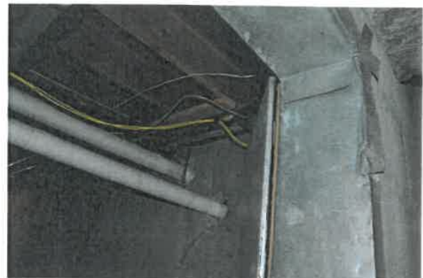
Figure 3-43 Access Door and Frame to Crawlspace in Basement Not Fire-Rated
