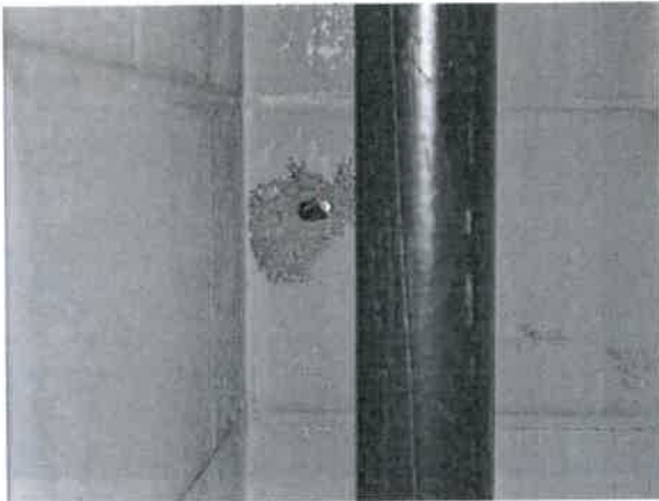
Figure 3-15 Unsealed Hole on the Concrete Wall of Smoke Room
