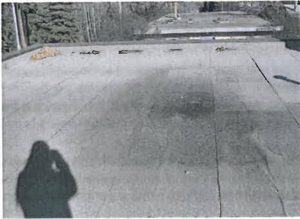
Figure 3-23 Water Ponding Deposits on Roof
