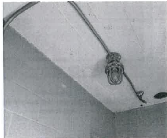
Figure 4-9 Viewing Other Side of Masonry Wall Within Oxygen Storage Room. No cracking visible.
