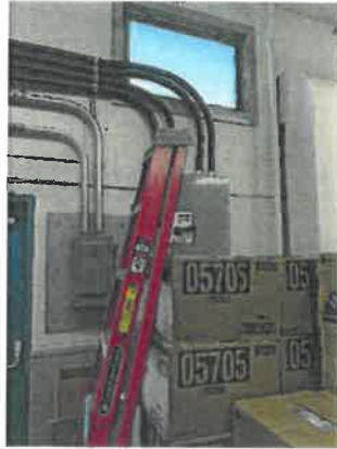
Figure 6-3 Insufficient Space in Front of Electrical Equipment
