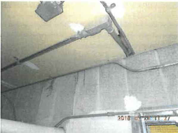
Figure 4-6 Staining on Interior Masonry Wall of Vault Room
