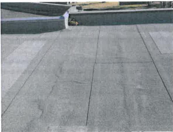
Figure 3-25 Blister Strips on the Roof
