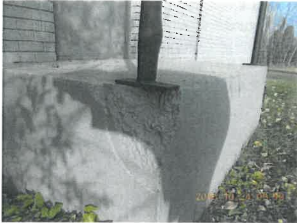
Figure 4-22 Viewing Damage to Concrete and Steel Column of East Apron
