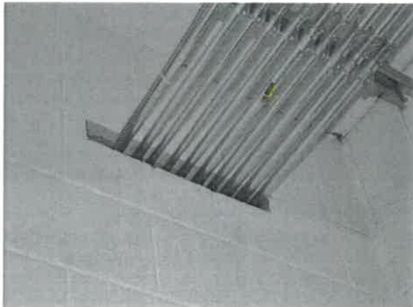
Figure 3-36 Conduits' Wall Penetrations Requiring Fire Sealant in Mechanical Room
