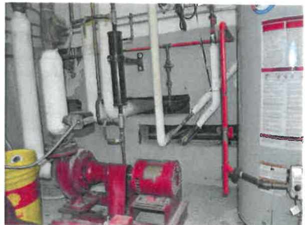
Figure 3-37 Pipe's Wall Penetrations Requiring Fire Stopping or Sealant
