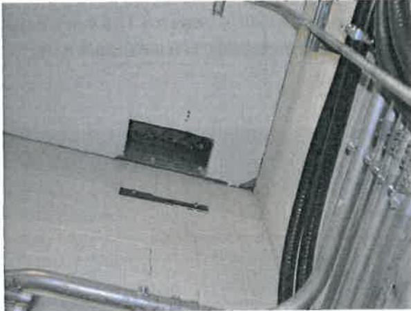
Figure 3-38 Opening on Ceiling Requiring Fire Sealant in Mechanical Room
