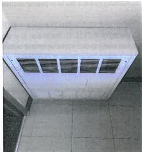
Figure 5-12 Force Flow Heater
