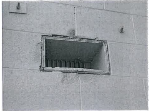
Figure 3-14 Unsealed Opening Around Louvre to Mechanical Room
