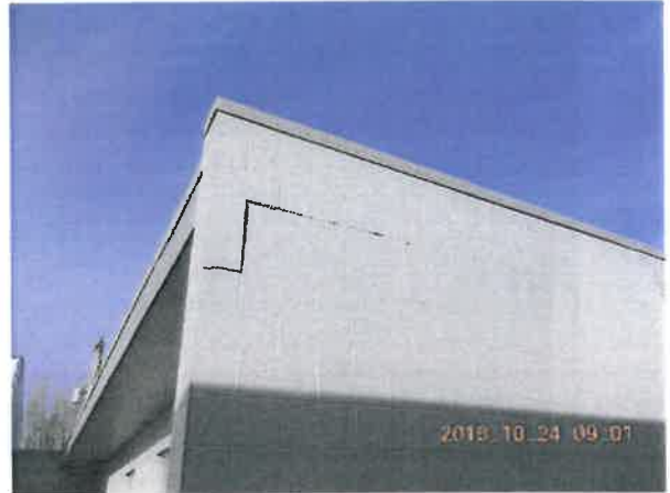
Figure 4-13 Viewing Horizontal Crack in Above Bond Beam at SE Corner of Chamber
