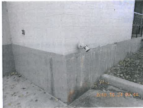
Figure 4-3 Viewing NW Face with Corrosion Staining
