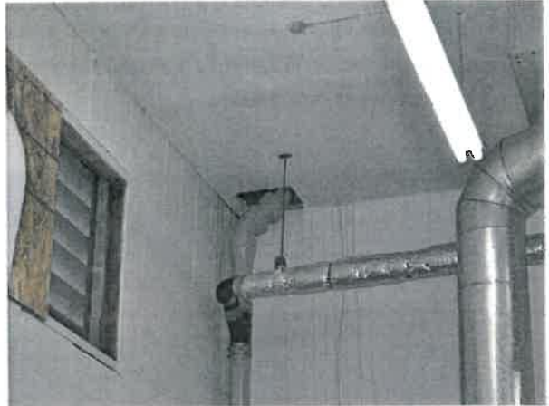
Figure 3-39 Pipe's Ceiling Penetration Requiring Fire Sealant in Mechanical Room
