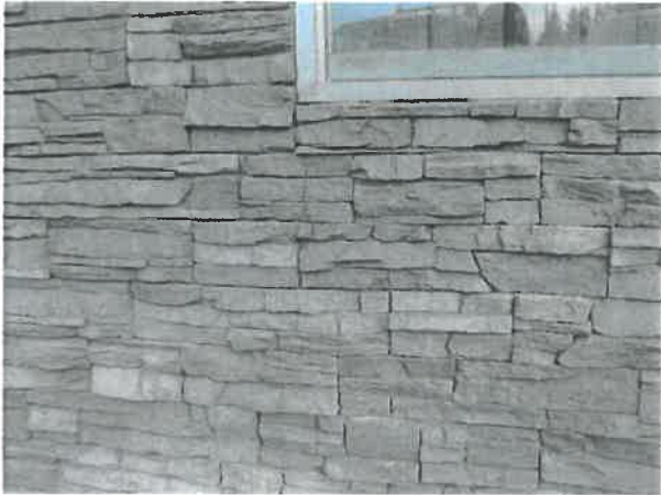
Figure 3-9 Cracks on Stone Veneer
