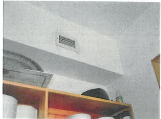
Figure 3-35 Vent in Janitor Room Not Fire-Stopped
