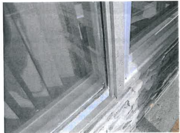
Figure 3-22 Broken Sealant at Bottom of Sealed Unit
