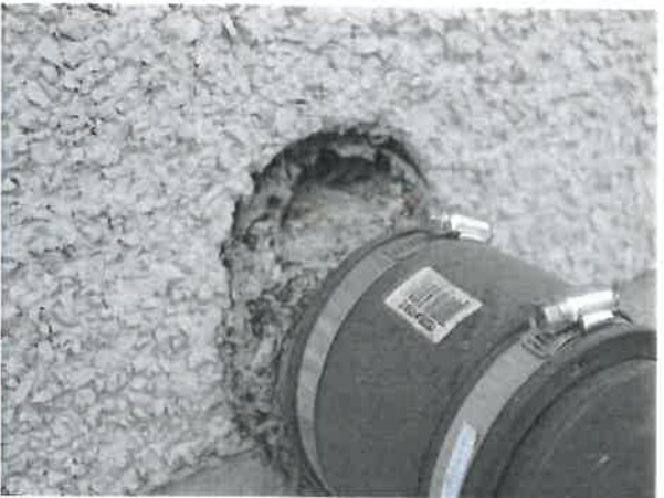
Figure 3-12 Unsealed Pipe Penetration
