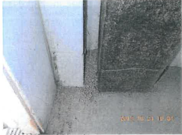
Figure 4-21 Potential Vermiculite Fill in Oxygen Storage Room
