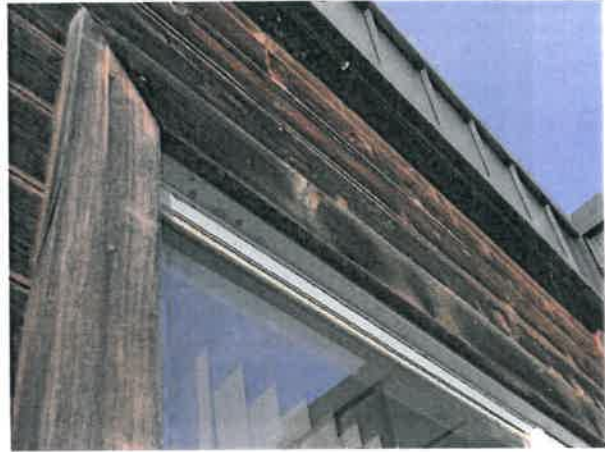
Figure 3-6 Missing Metal Head Flashing Above Window Trim
