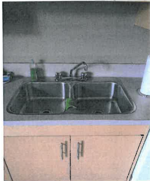
Figure 5-4 Double Compartment Sink
