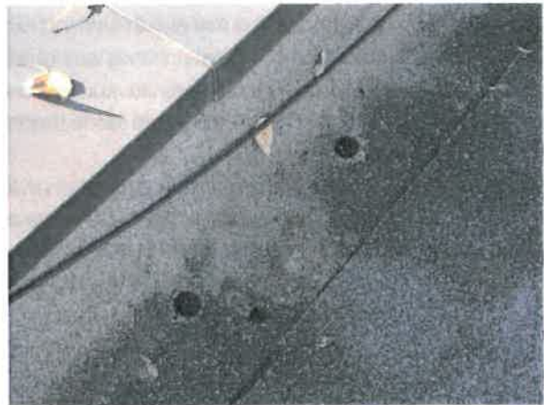
Figure 3-26 Moss at the Parapet Base on the Roof
