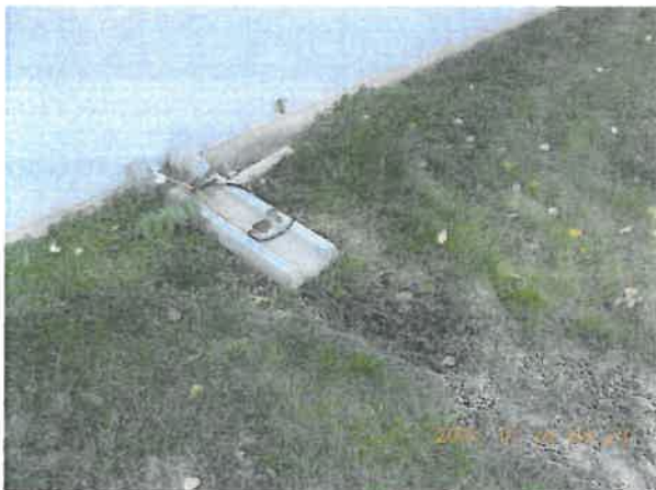
Figure 2-5 Viewing Scour at North Roof Drain Location
