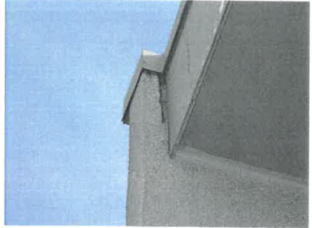
Figure 3-2 Missing Stucco at Fascia to Wall Location
