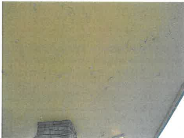
Figure 3-29 Paint Blister on Soffit of the Main Entrance Canopy
