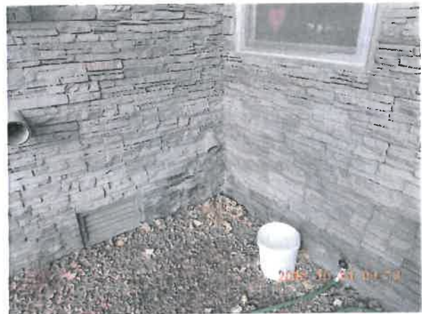
Figure 2-2 Missing Splash Pad Under Roof Drain Near Main Entrance
