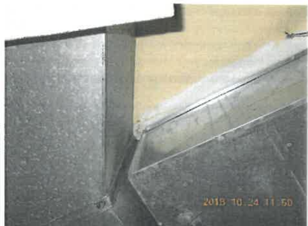
Figure 4-7 Viewing Staining on Drywall Ceiling Above Ductwork
