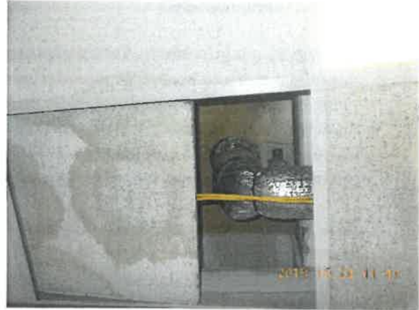
Figure 4-5 Example of Leak at Roof Drain Location
