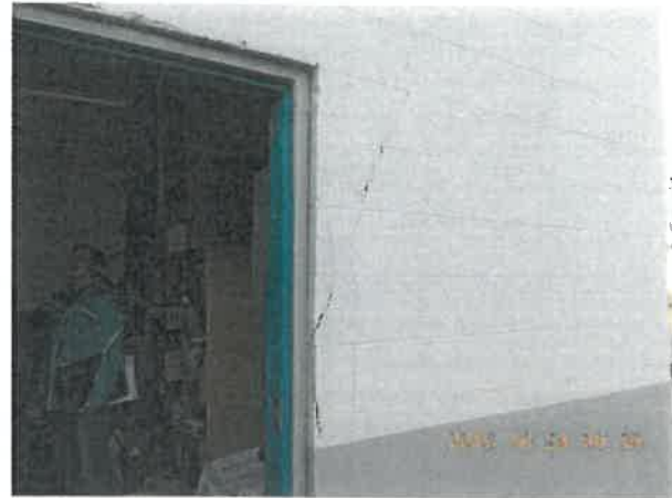
Figure 4-17 Viewing Severe Crack Near Door in North Wall
