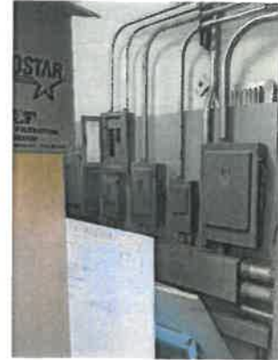
Figure 6-4 Insufficient Space in Front of Electrical Equipment
