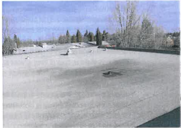
Figure 3-24 Water Ponding Deposit Around Roof Drain
