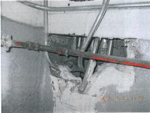
Figure 4-20 Viewing Vermiculite Fill at Conduit Penetration Into Masonry Wall Within Boiler Room at the SE Corner
