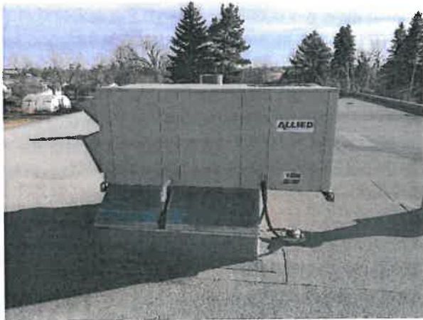
Figure 5-13 Roof Top Unit
