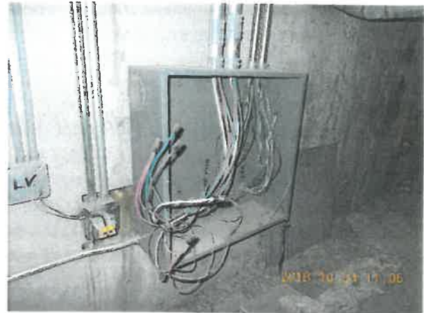
Figure 6-10 JB Cover Missing
