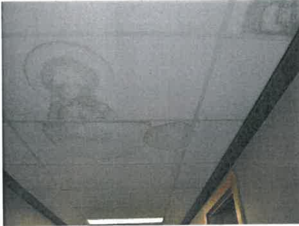
Figure 3-32 Water Stain on Ceiling Tiles Over Corridor
