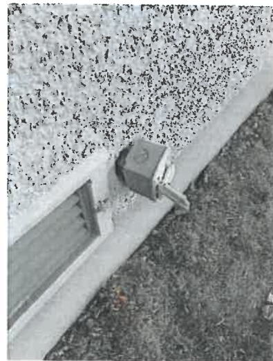
Figure 6-6 Damaged Exterior Receptacle
