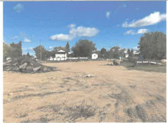
Ardmore staging area out of commission with new storm sewer work being done.
