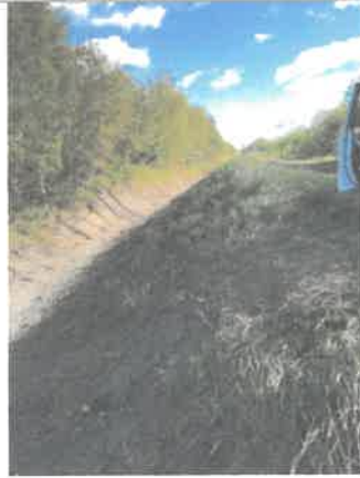
M.D. of Bonnyville cleaned side of trail to alleviate flooding on ALO property.
