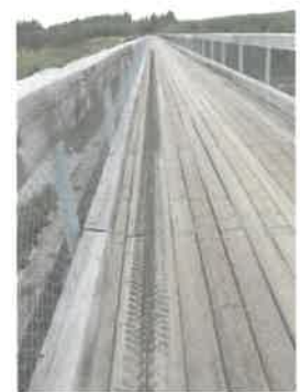
Burnt out marks on the trestle from a vehicle.
