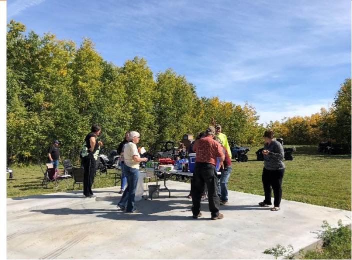
Installation of cement pad at Abilene Junction. Trail volunteers celebrated with a ride and wiener roast.
