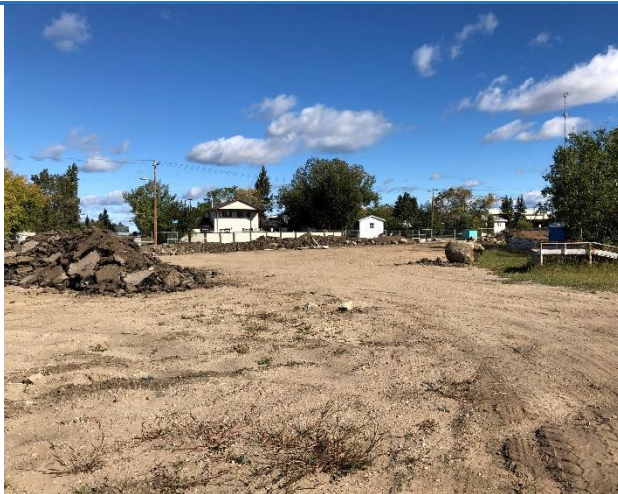
M.D. installing drainage ditch in Ardmore and using the staging area as a construction zone.
