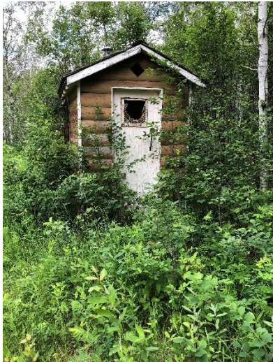
Bear damage / overgrown
