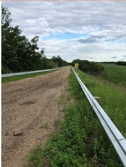
Guard rails at Ashmont buried trestle – installed by County of St. Paul as part of the water line construction.
