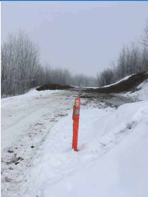
Issue north of Smoky Lake with water from a spring opened during water line construction
