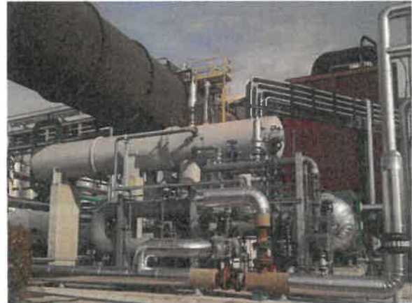
Figure 24 – ORC System (8 MW)
