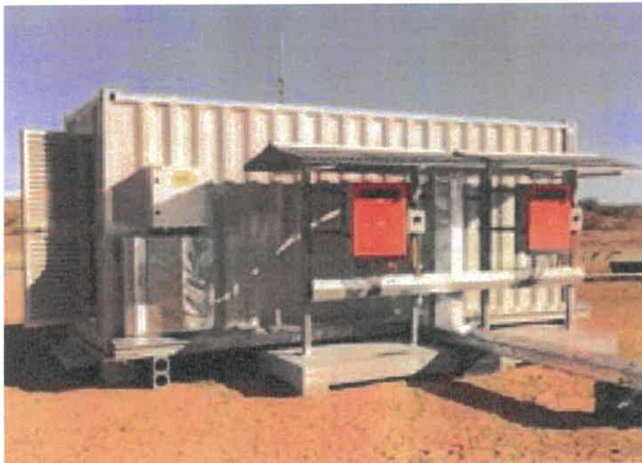
Figure 19: Battery Storage Module
