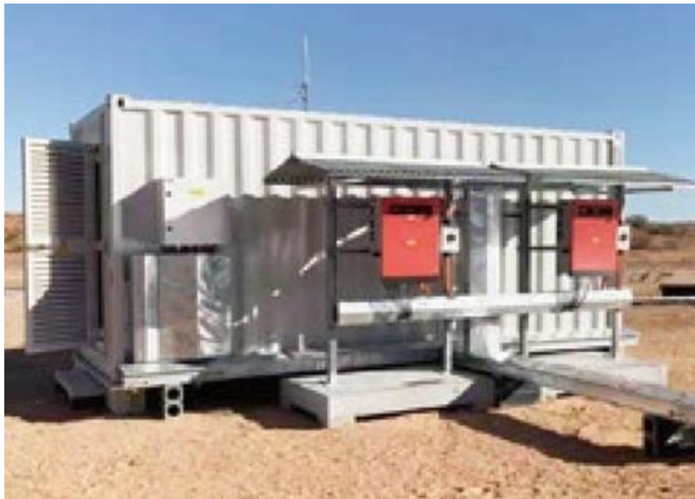
Figure 19: Battery Storage Module
