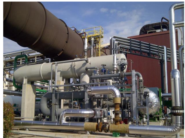
Figure 24 – ORC System (8 MW)
