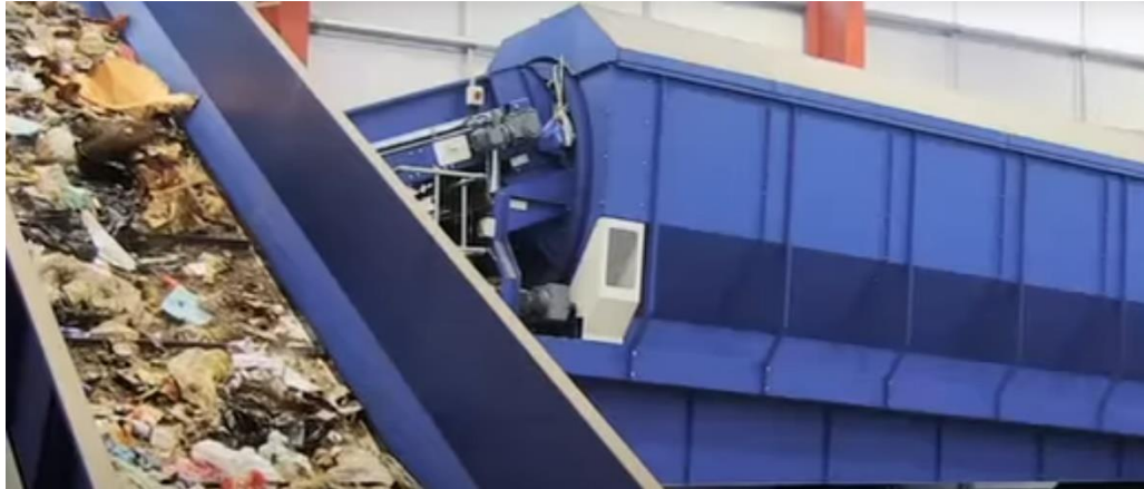
Figure 3: Conveyor to Trommel
