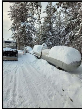
Photo 8 – Two aboveground propane tanks for main household.
