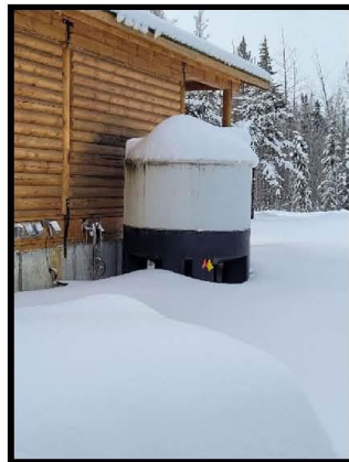
Photo 26 – Entertainment lodge’s water tank, facing southwest.
