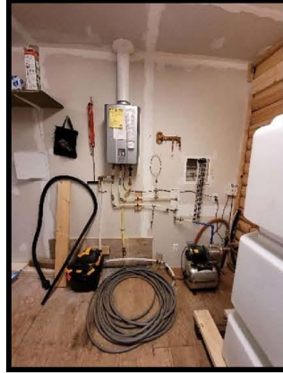
Photo 29 – Entertainment lodge mechanical room.
