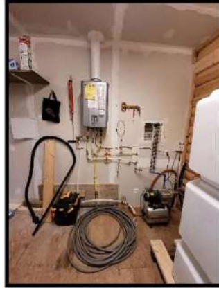
Photo 29 – Entertainment lodge mechanical room.
