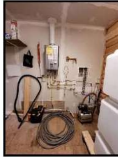
Photo 29 – Entertainment lodge mechanical room.
