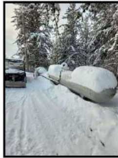
Photo 8 – Two aboveground propane tanks for main household.
