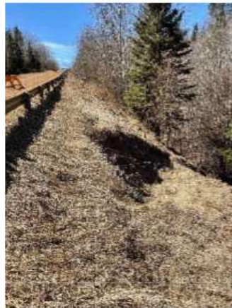
Photo 1: Slump in the embankment
