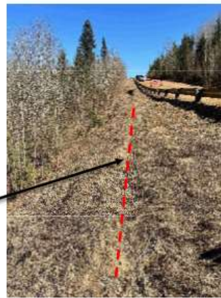
Photo 2: Head scarp along the embankment
