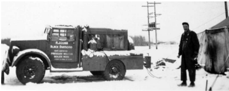
Figure 25. Welding truck constructing two 8-inch lines from Nisku to Devon Field, Leduc, Alberta, circa 1947. Credit: Glenbow Archives / PA-3027-8.
