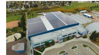
Camrose Rec Centre Solar Array
