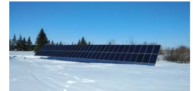
Solar Array in Camrose County
