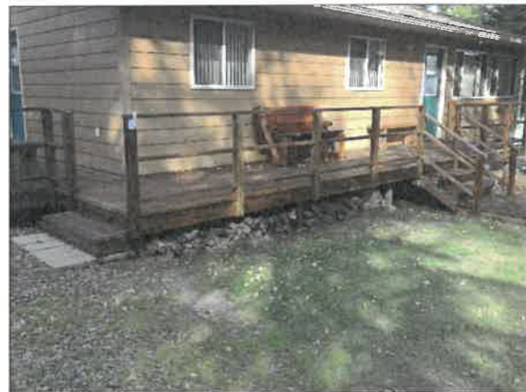
Combustible Siding and Deck Construction
