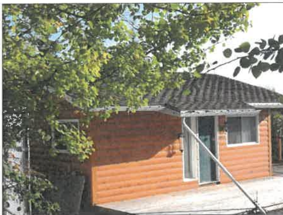
Combustible Old-Curled Asphalt-Shingle Roof
