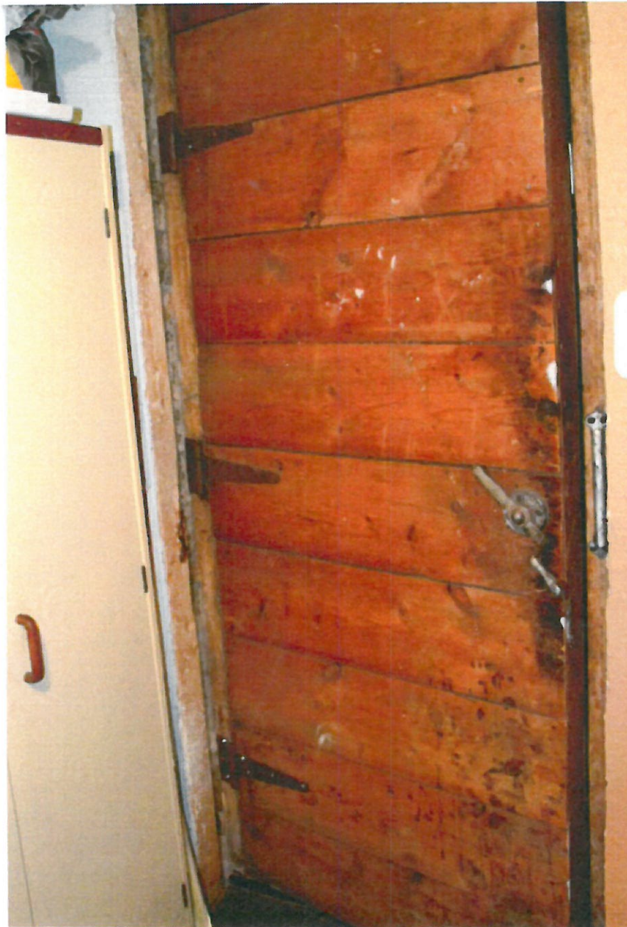
Cold storage door and hardware
